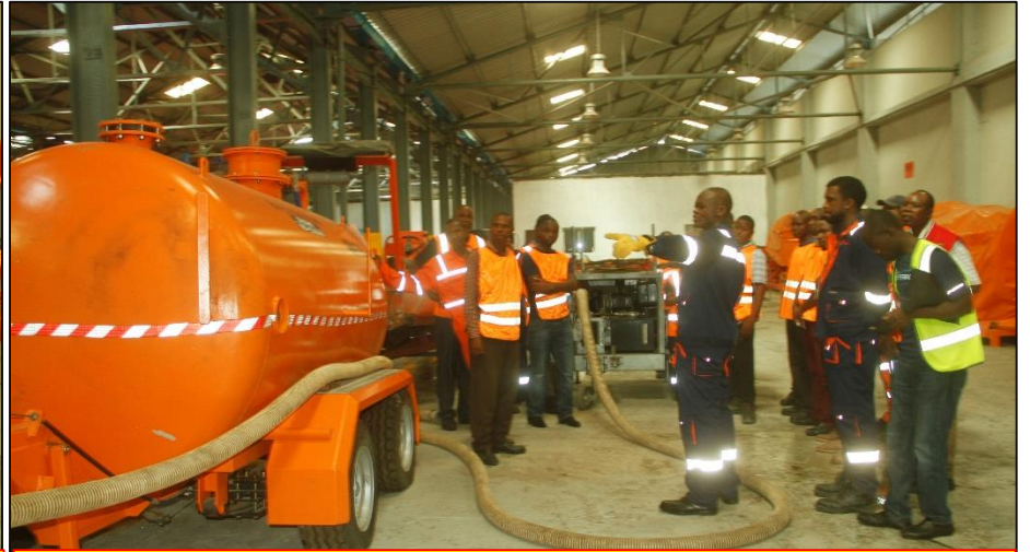
Engr Okanga explains the functionality of a recovered oil storage tank and its connections to the vacuum recovery unit
